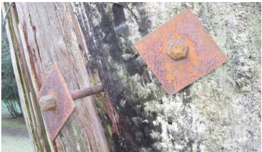
Photo 3: Steel washers and bolts no longer effective
